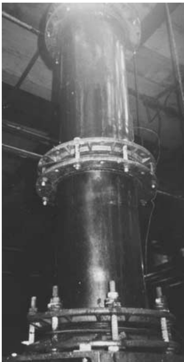
Figure 8: Glass Section of 8-inch Line to Condenser
