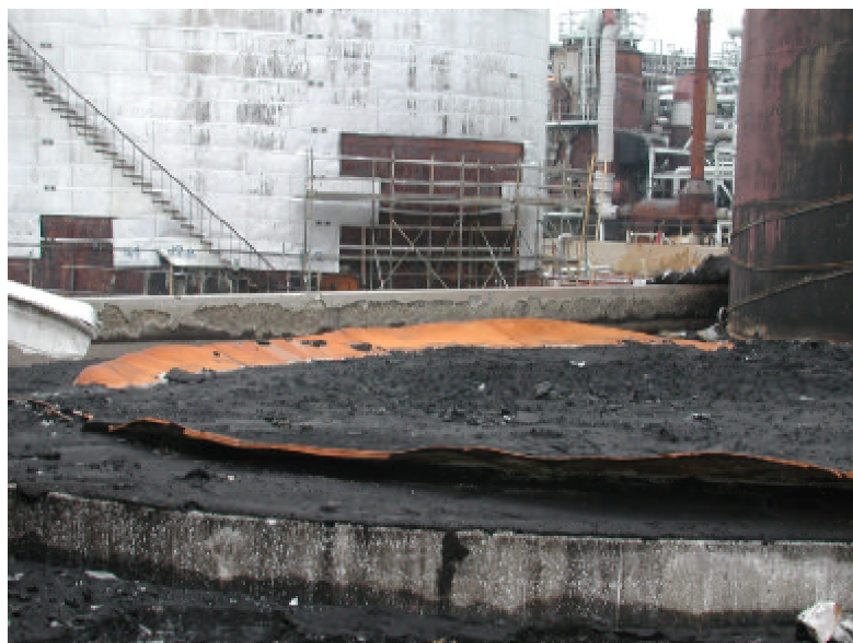
Figure 8. Floor of tank 393 showing uplift due to internal deflagration (before separation of shell).
