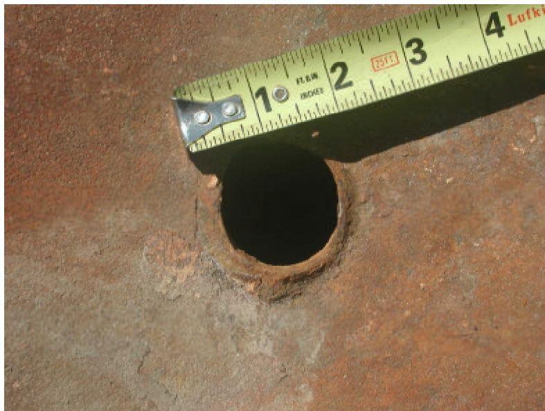
Figure 6. Hole in roof of tank 393 through which temporary hose was inserted.
