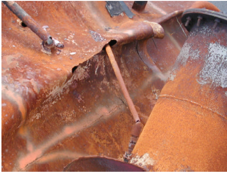
Figure 5. Elongated hole on roof of tank 393 (covered by insulation at time of incident).
