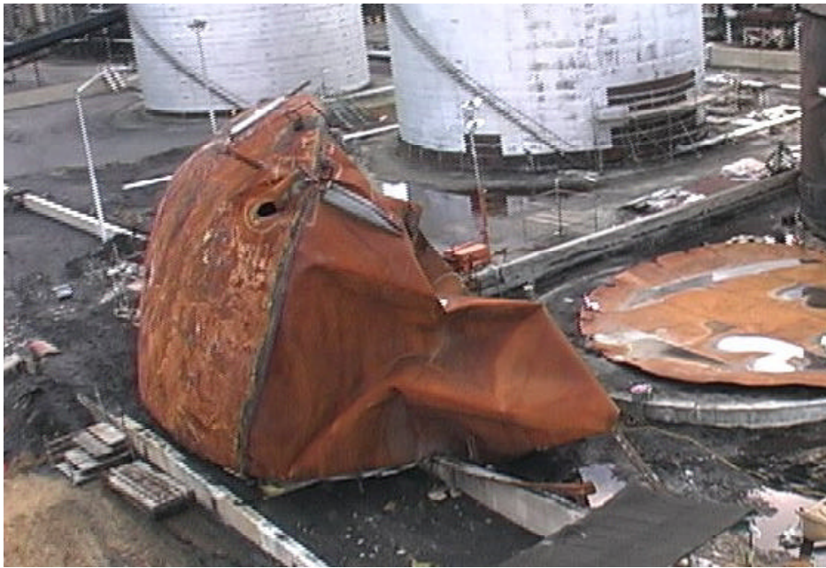
Figure 2. Tank 393, collapsed at northeast corner of storage tank dike. (Note floor of tank 393 to the right of tank shell.)
