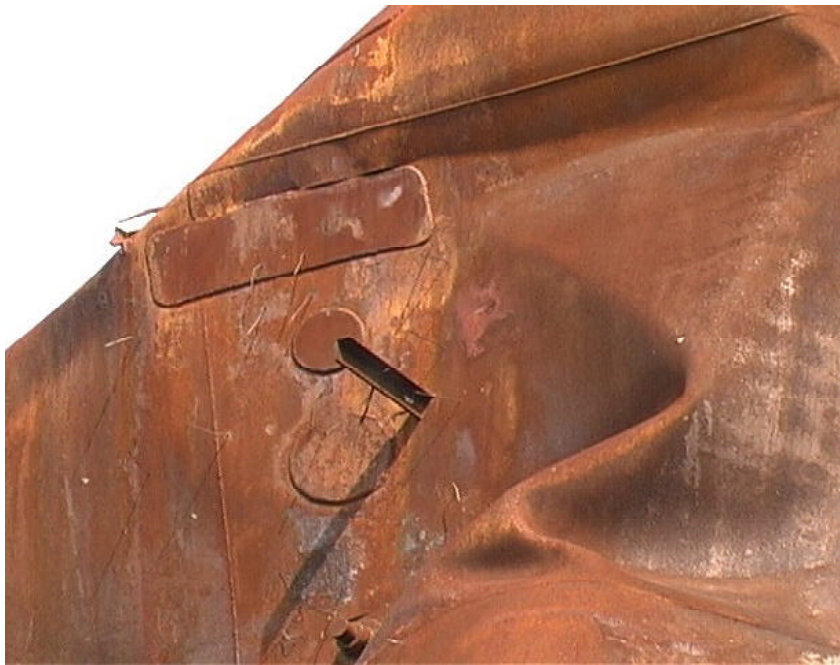
Figure 4. Side of tank 393 showing series of patches.
