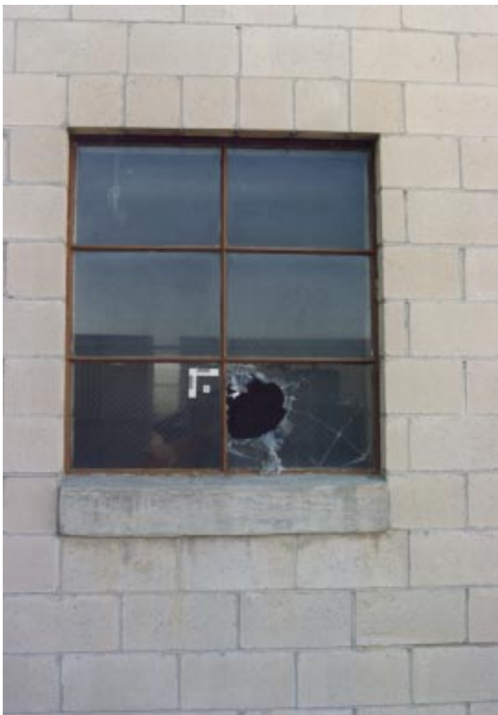
Exhibit 2-4. Broken Window, South Side
