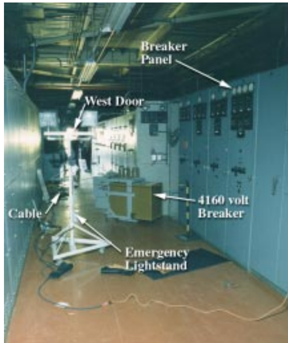
Exhibit 2-2. Switchgear Looking West Toward Exit Door
