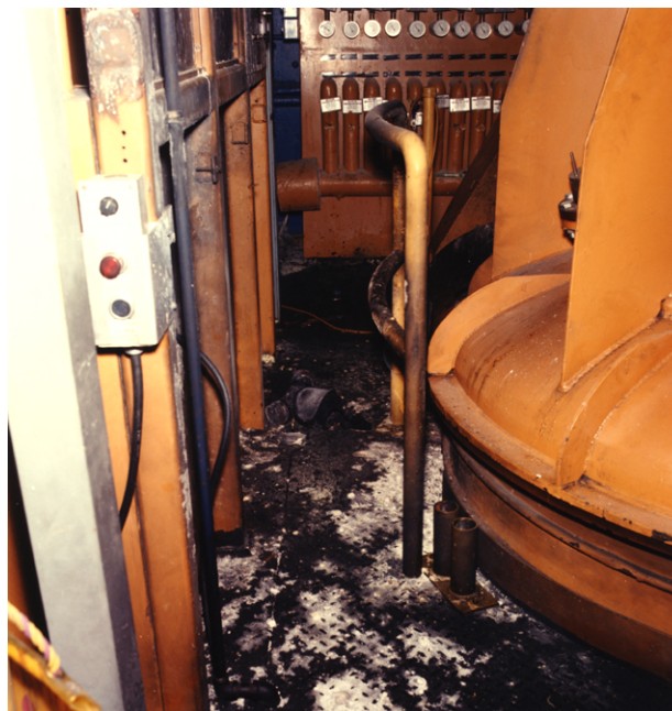
Exhibit #7. Residual NaK from Explosion Near Furnace
