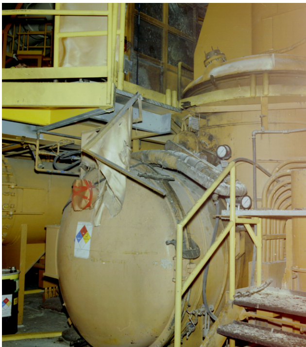
Exhibit #8. Furnace Showing Explosion Damage
