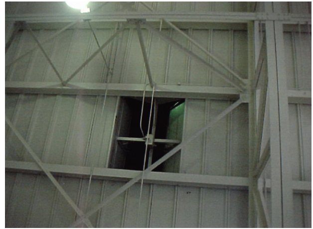
Exhibit #14. Open Roof Vents
