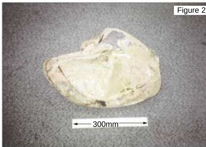
Base of hot water cylinder
